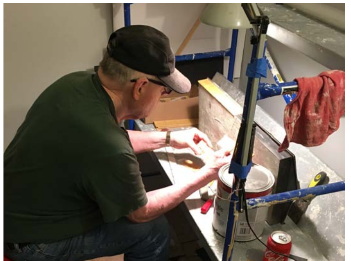
Above. Dick sealed the bottom of the structure with white paint before adding the pre-painted DPM sides.
