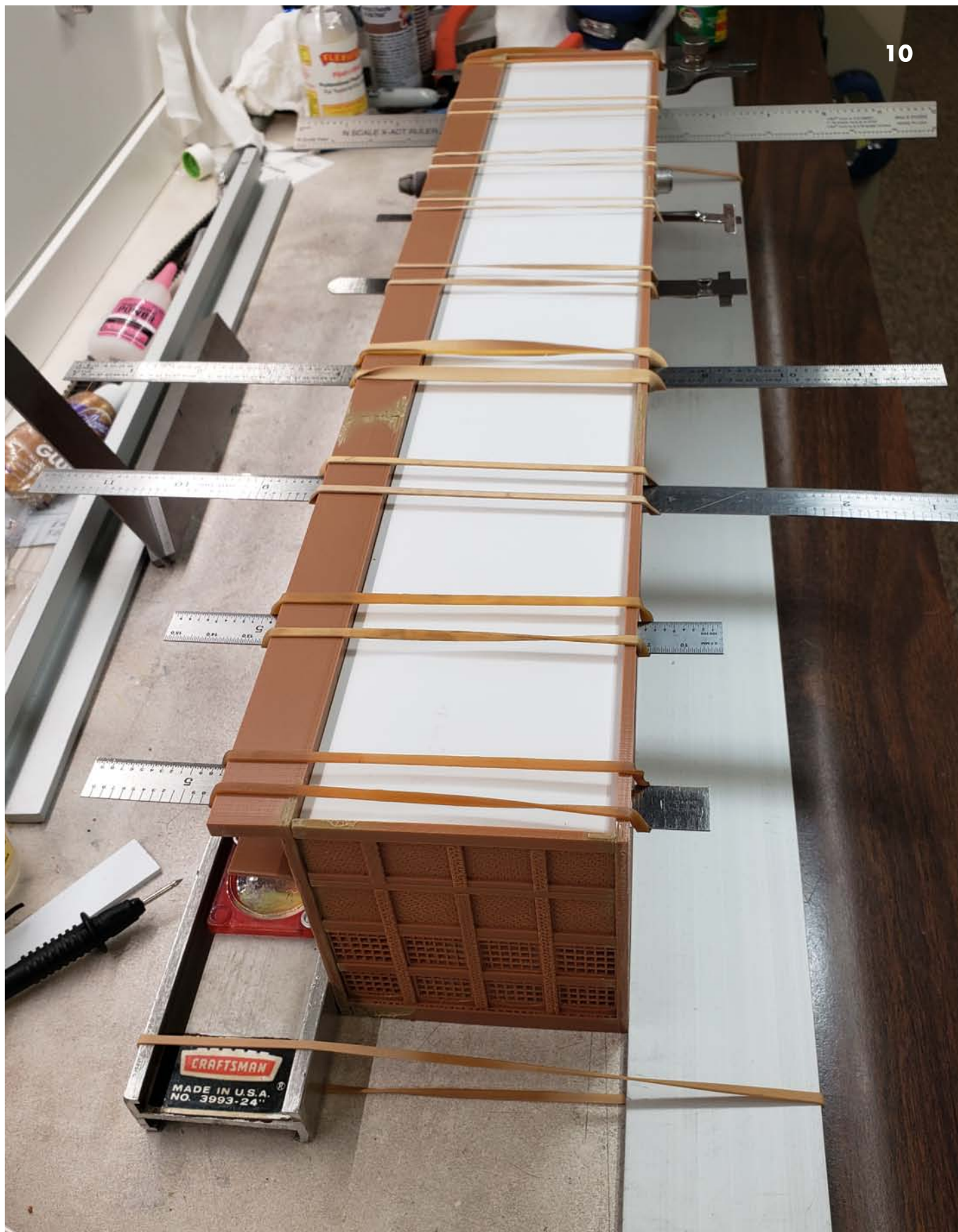
Image 10. I used an aluminum level and a piece of aluminum stock to keep the sides at the top of the building to straight.
