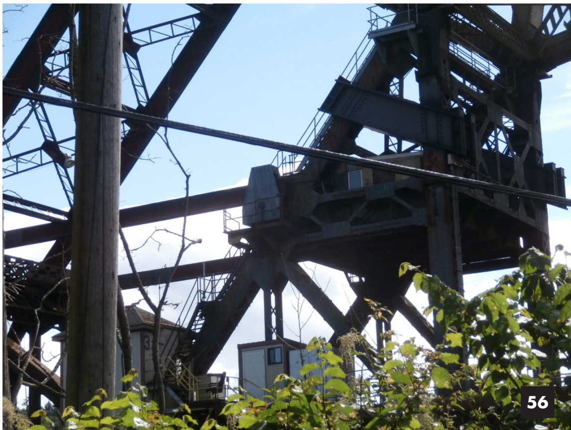
Image 56: Looking at the lifting mechanism shack on the north tower from the east side. The two horizontal bars are the operating arms. Trains pass directly under the lifting mechanism shack.
