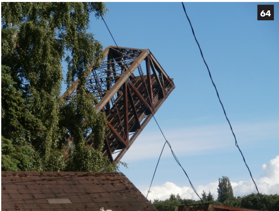
Image 64: View of the lifting span looking south from Seaview Ave NW. The bridge was raised while I was walking under the tracks.
