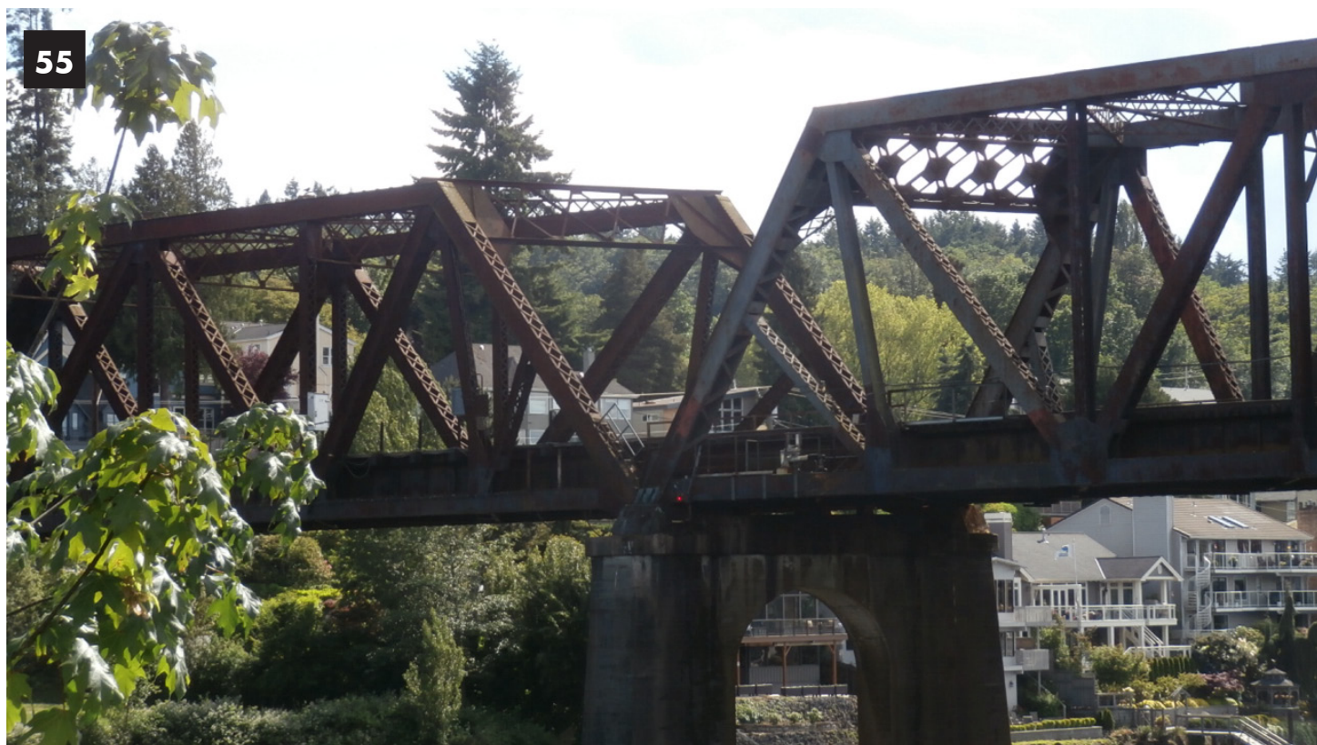
Image 55: The bridge is lowered. Looking southwest the fixed span is on the far side of the bay. The lifting span is to the right.
