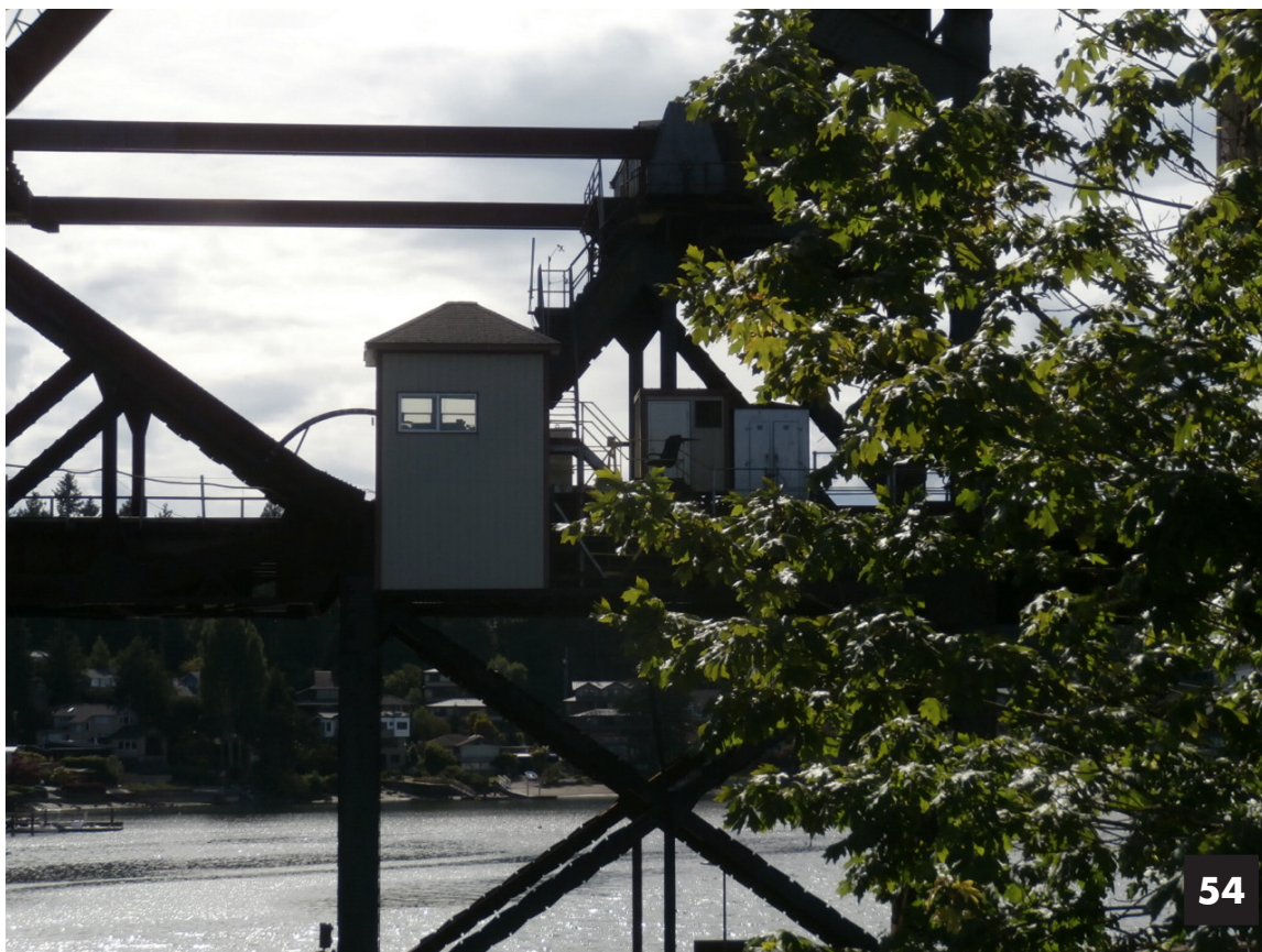
Image 54: A closer look at the operator's shack from June, 2017. At this date the exterior has been updated and the window arrangement changed from the 1950s configuration.
